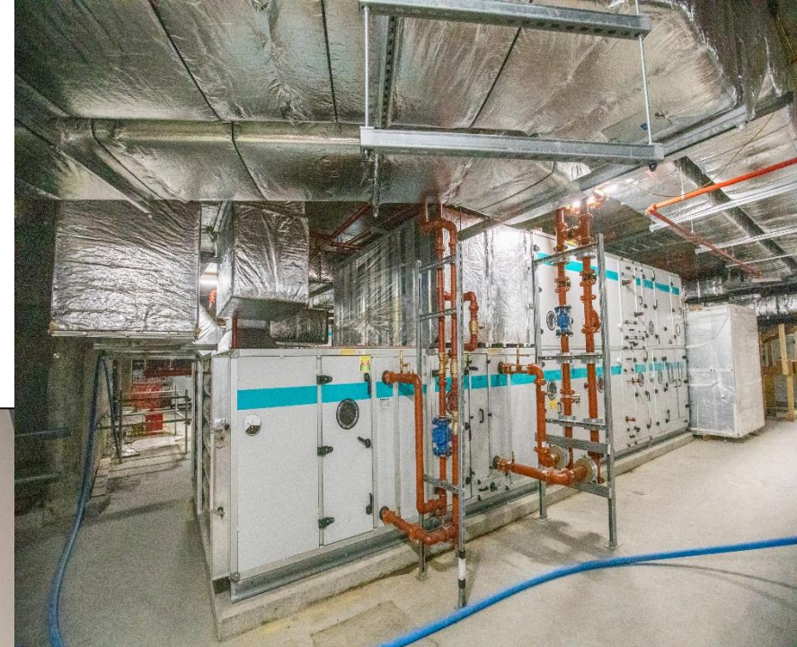
Air Cooling Handling Units
